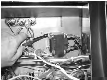
Express Filter Transformer
