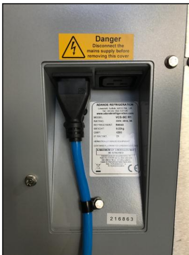
Figure 3: Mains connection point
